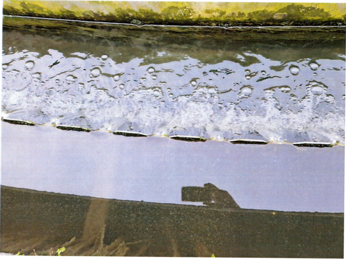
Photograph 3: View of Clarifier no. 1 at Ennis North Waste Water Treatment Plant (D0048-01)
