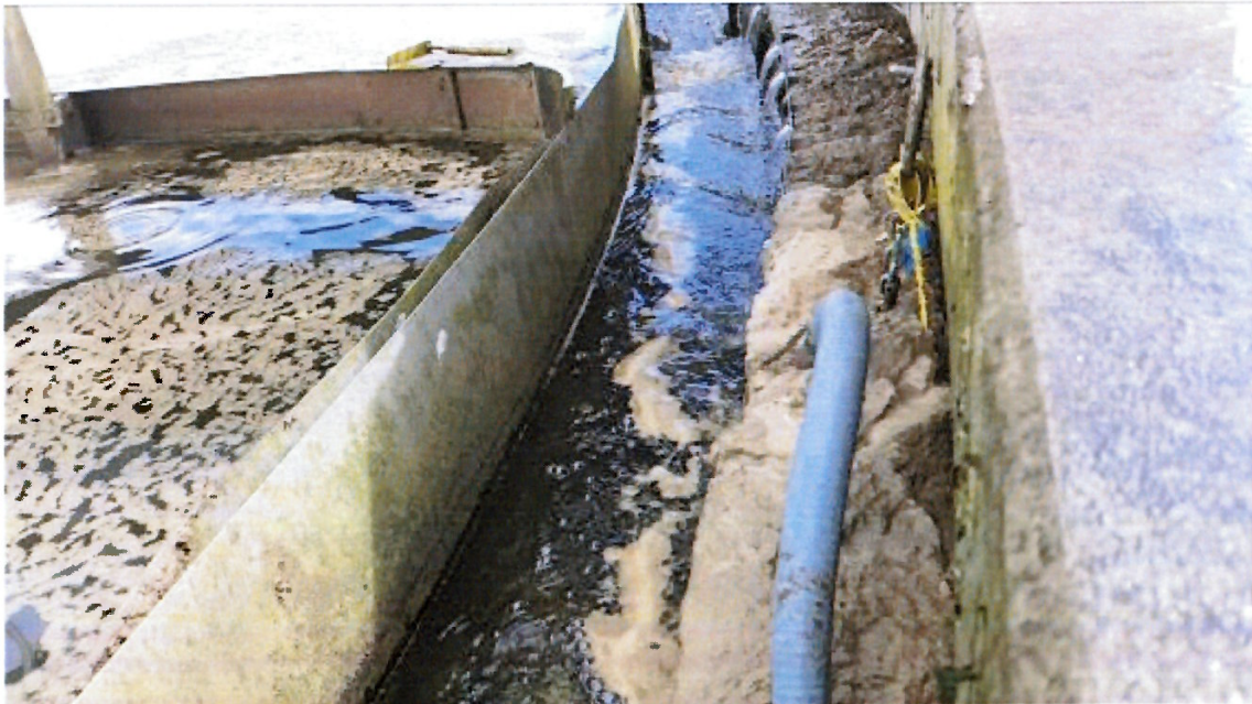
Photograph 2: Sludge carryover observed in clarifier No. 1.
